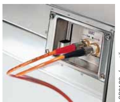
Fig. 5/36 View from below showing system interface (SCADA) with FO connection (for remote communications)
